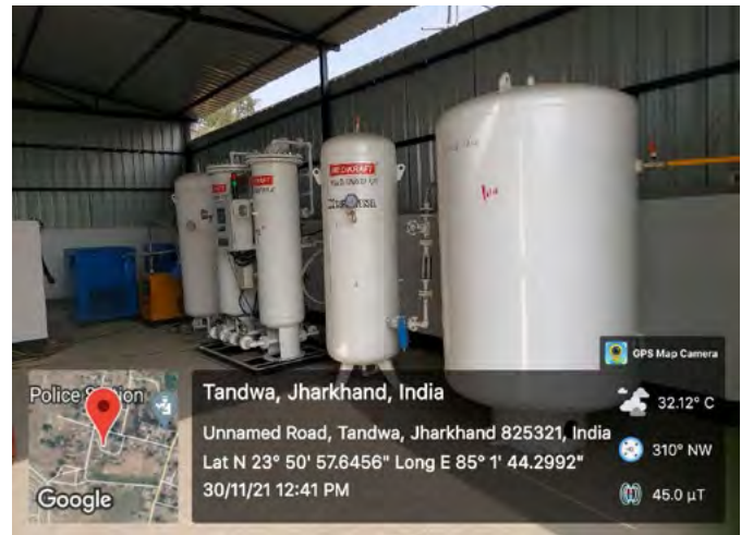
Oxygen Plant Chatra
