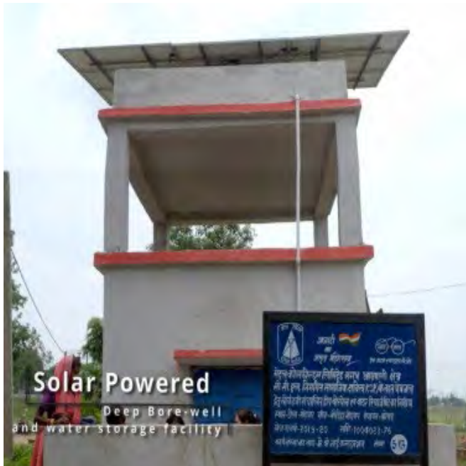
Solar Power operated Deep Bore well
