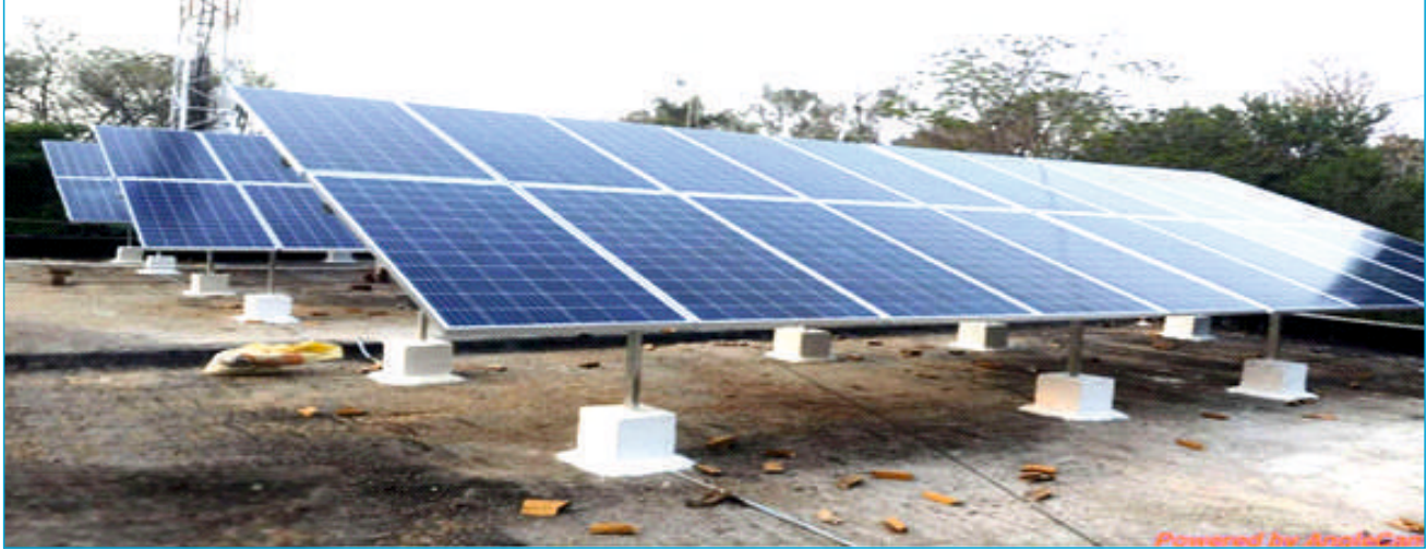
Solar panel at CCWO, office
