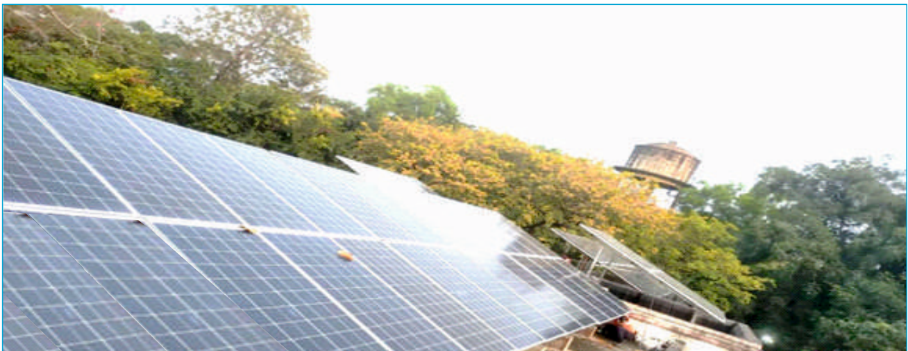
Solar Panel at Jagjivan Nagar Guest House
