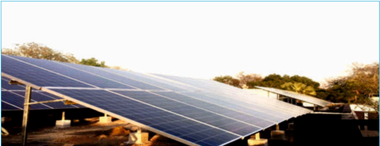
Solar Panel at Nursing Hostel
