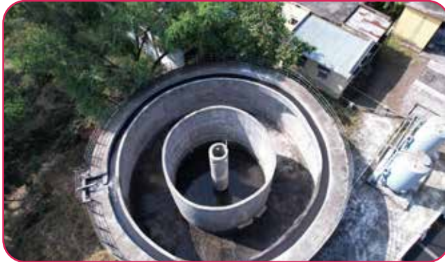
Mine Water Treatment Plant at Sohagpur Area
